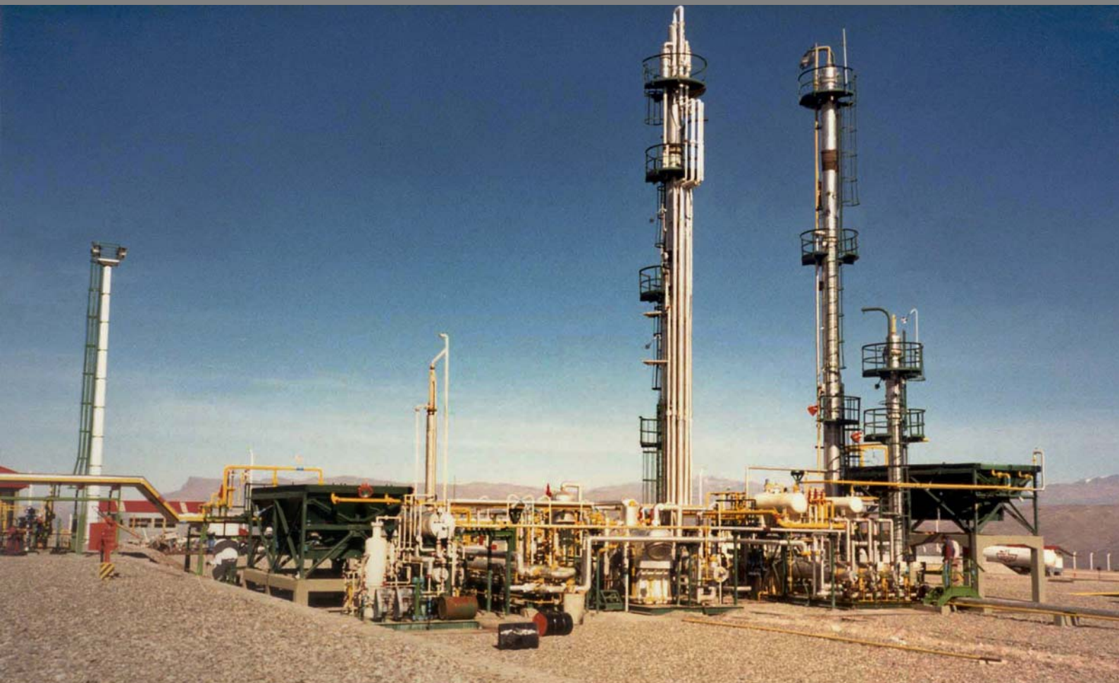
GAS TREATMENT PLANT - PETROZUATA - SAN DIEGO DE CABRUTICA, VENEZUELA - UNIVERSAL COMPRESSION (THROUGH VEN-TECNA)
