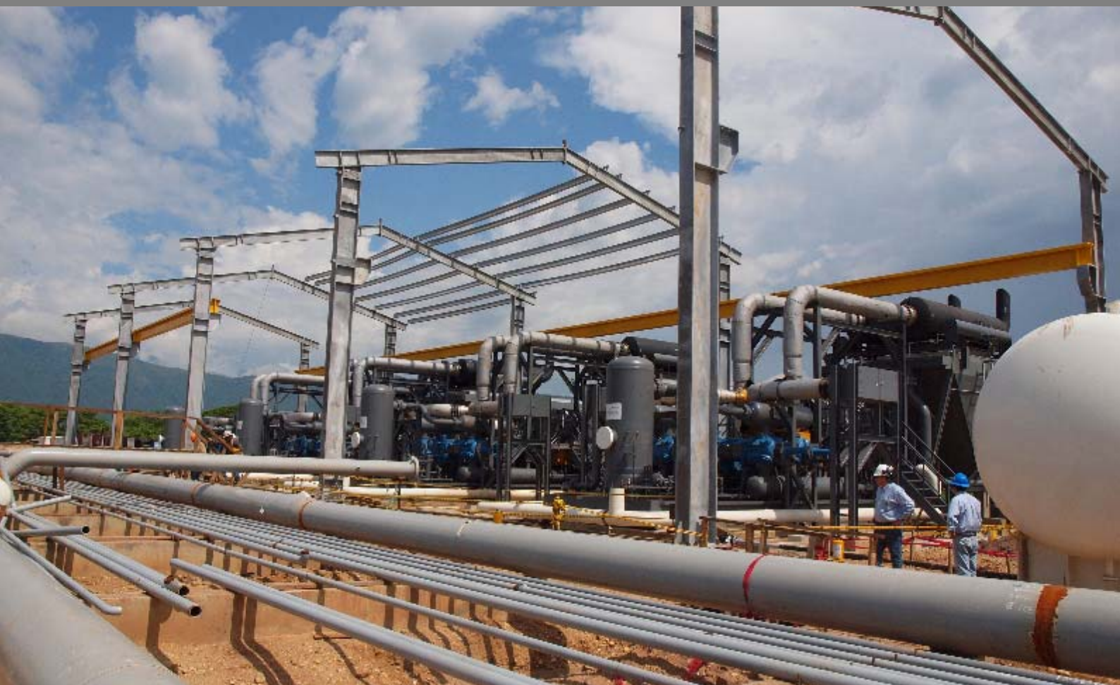
GAS COMPRESSION PLANTS – JAGUA DEL PILAR, CURUMANÍ, SAN ALBERTO AND PUENTE GUILLERMO – BALLENA – BARRANCA BERMEJA GAS PIPELINE, COLOMBIA – TGI
